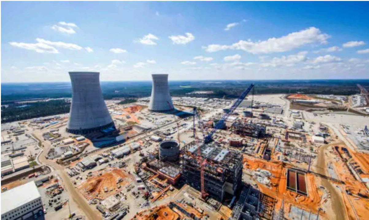
Nuclear power plant Vogtle Unit 3 and 4 sites are under construction near Waynesboro, Ga., in February 2017. Georgia Power/Handout via Reuters
