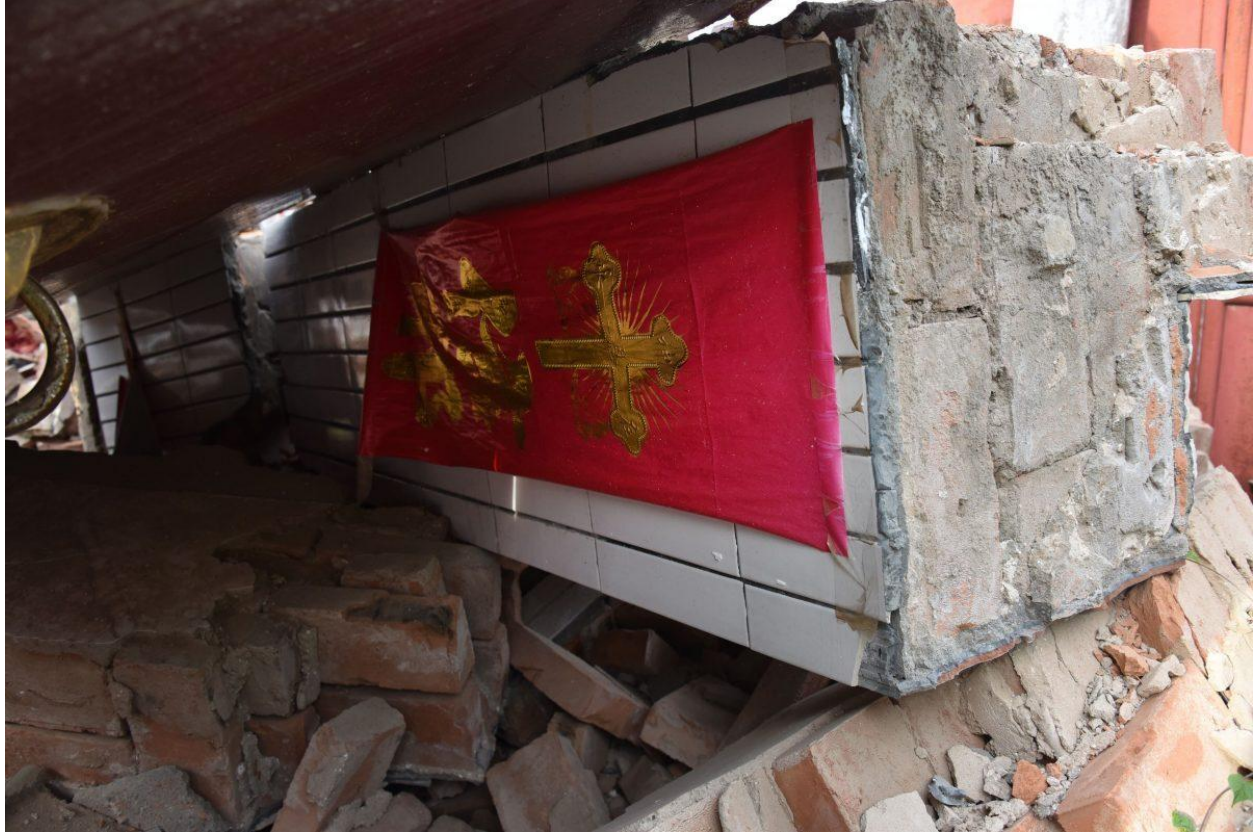
The pillar of a demolished Catholic church is seen in Puyang, in China's central Henan Province on Aug. 13, 2018. (Greg Baker/AFP/Getty Images)
