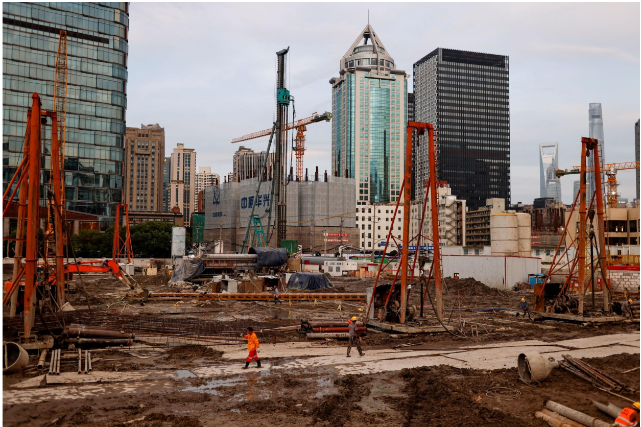
Workers labor at a construction site in Shanghai, China on July 12, 2021. (Aly Song/Reuters)
